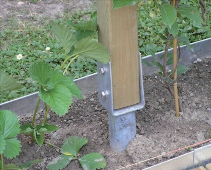
Plant support post fixation
